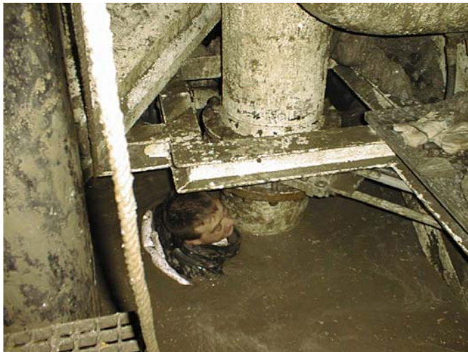
Figure 3. Repair works on stone crusher, personnel standing within bentonite slurry (4 th Elbe tunnel)
