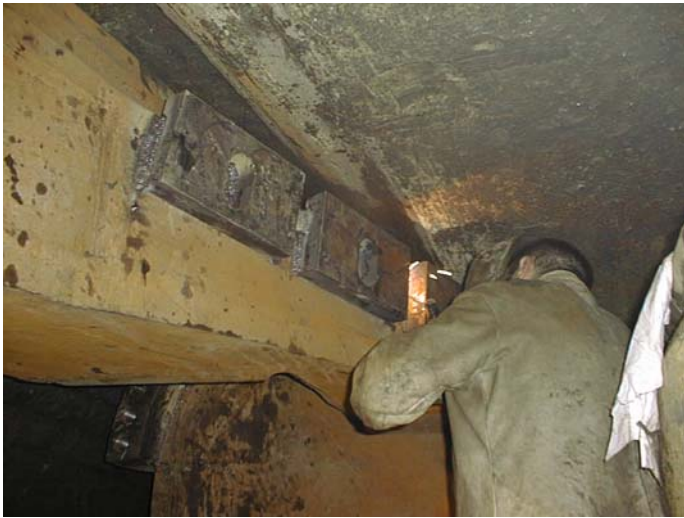
Figure 2. Welding for repair works due to excessive wear on backside of cutterhead (4 th Elbe tunnel)
