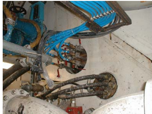
Figure 5. Special flanged connections installed at the bulkhead to allow manned interventions to be carried out in the bentonite.
