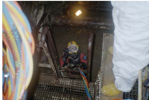
Figure 7. Use of divers for maintenance and repair work in the working chamber.
