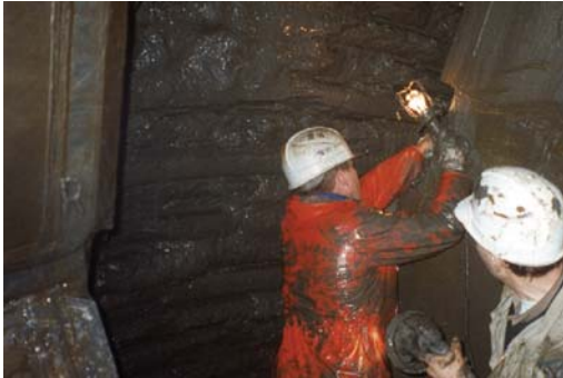
Figure 4. Soft rock tunnel face – tool change at 3.5 bar at the 4th tube Elbe Tunnel (Hamburg, Germany).
